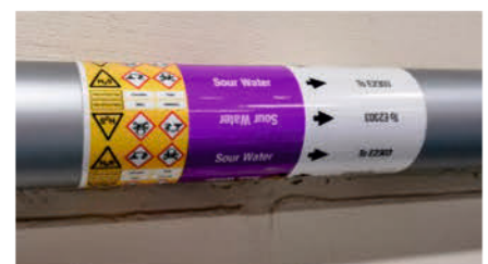
Pipe Marking according ISO 20560-1
